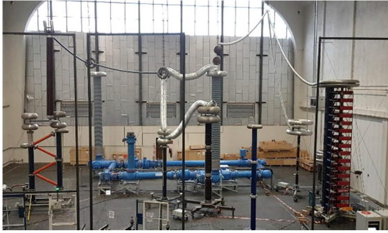
Figure 7 HVDC GIS with test setup for long-term test
